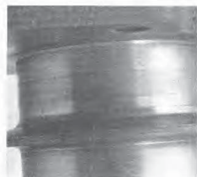
20.7 If the seals have worn grooves in the crankshaft journals, or if the seal contact surfaces are nicked or scratched, the new seals will leak
