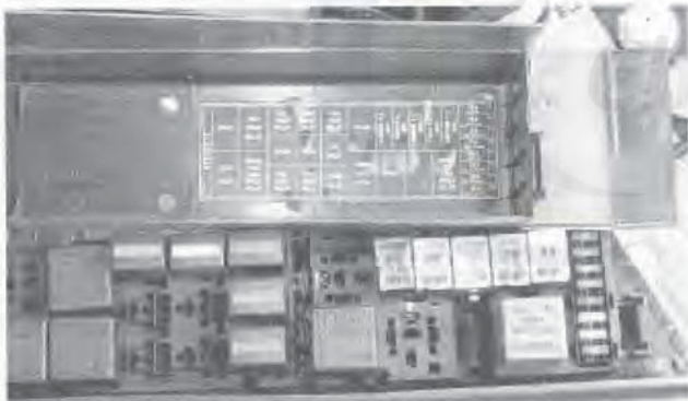
4.2 The relay for the engine cooling fans is located in the relay centre in the engine compartment
